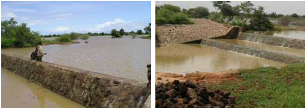
Figure 35. a) Water in water-spreading weir; b) Water-spreading weir in Kalfou (Tahoua region, Niger) (Photos: GIZ/Aboubacar Mounkaila).
