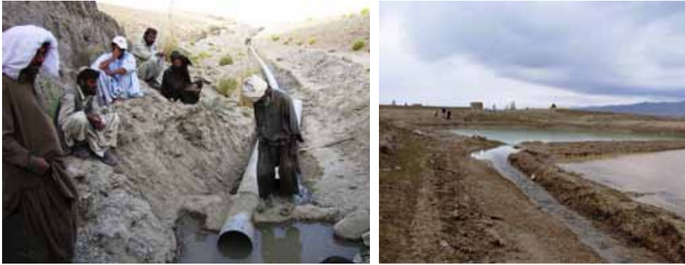
Figure 22. a) Villagers taking rest during improvement of the Qilla Iskan Khan karez system. They are installing a 30 cm wide PVC infiltration pipe inside the karez; b) The constructed geo-membrane reservoir (Photo: IUCN Pakistan, 2011 and 2010).
