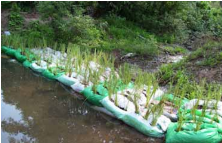
Figure 17. Example of check dam, Thailand (Photo: Hydro and Agro Informatics Institute (HAI), Bangkok)
