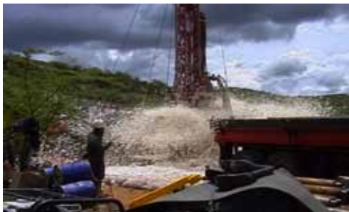
Figure 24. Drilling of deep boreholes, to increase access to a larger volume of stored groundwater reserves.
