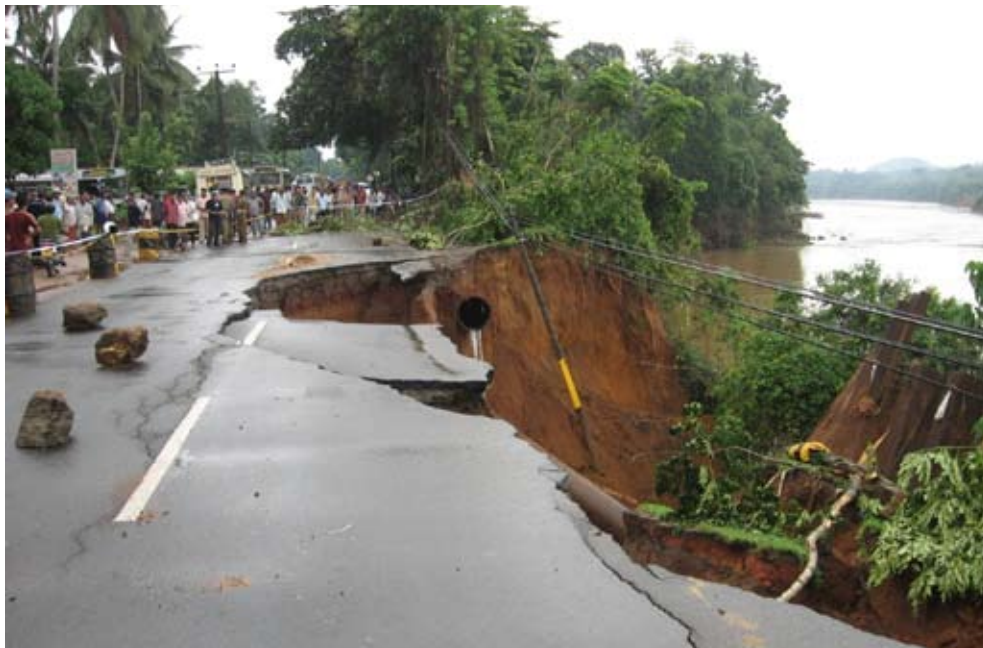
Figure 1: Kelani river bank erosion due to sand mining. A domestic water supply pipe line underneath the road got damaged and city water supply got disturbed for several days. (Photo: Badra Kamaladasa, Irrigation Department of Sri Lanka)
