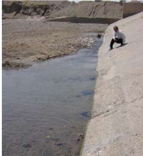
Figure 3: Water emerging from weepholes
