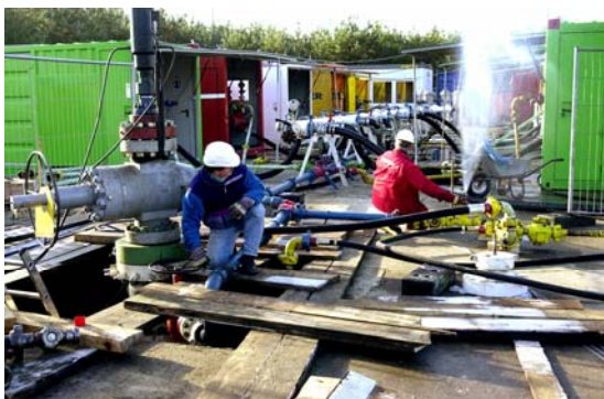
Figure 3: Impression from the stimulation experiments: wellhead with riser in front, ten high pressure pumps (HT400) with low and high pressure manifold in the back (photo by A. Weitze).
