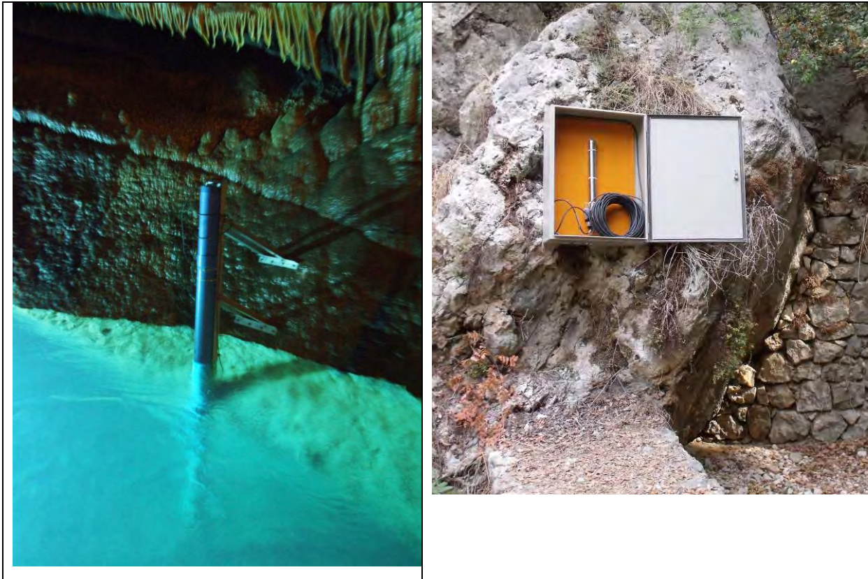
Figure 41: Multiparameter probe Troll 9500 installed in Jeita
