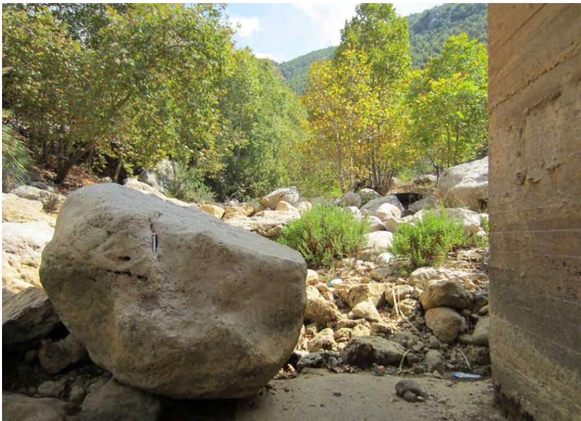
Figure A4: Boulder on top of basement structure at the bridge of Nahr es Zirghaya
