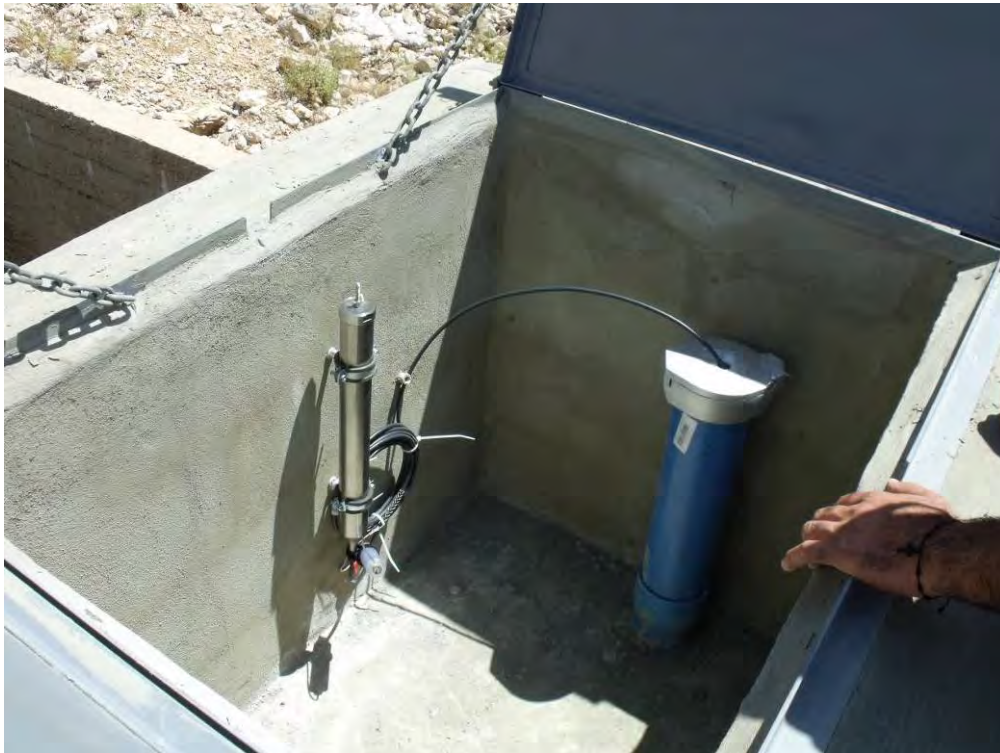
Figure 63: Head of PVC casing in concrete box with perforated hole for vented cable of multiparameter probe, connected to COM 300 unit for telemetric data transfer
