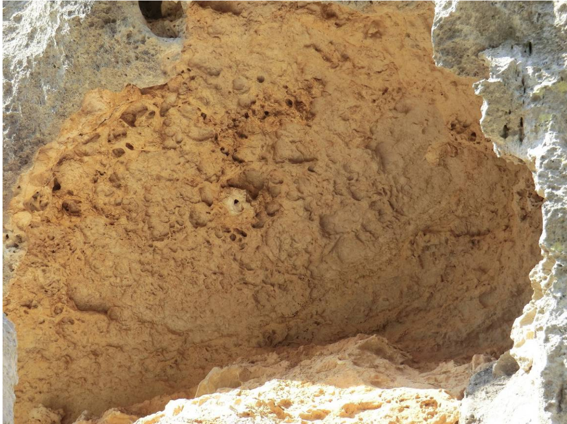
Figure 37: Detail showing the Cavity from Figure 36 (WP67)
