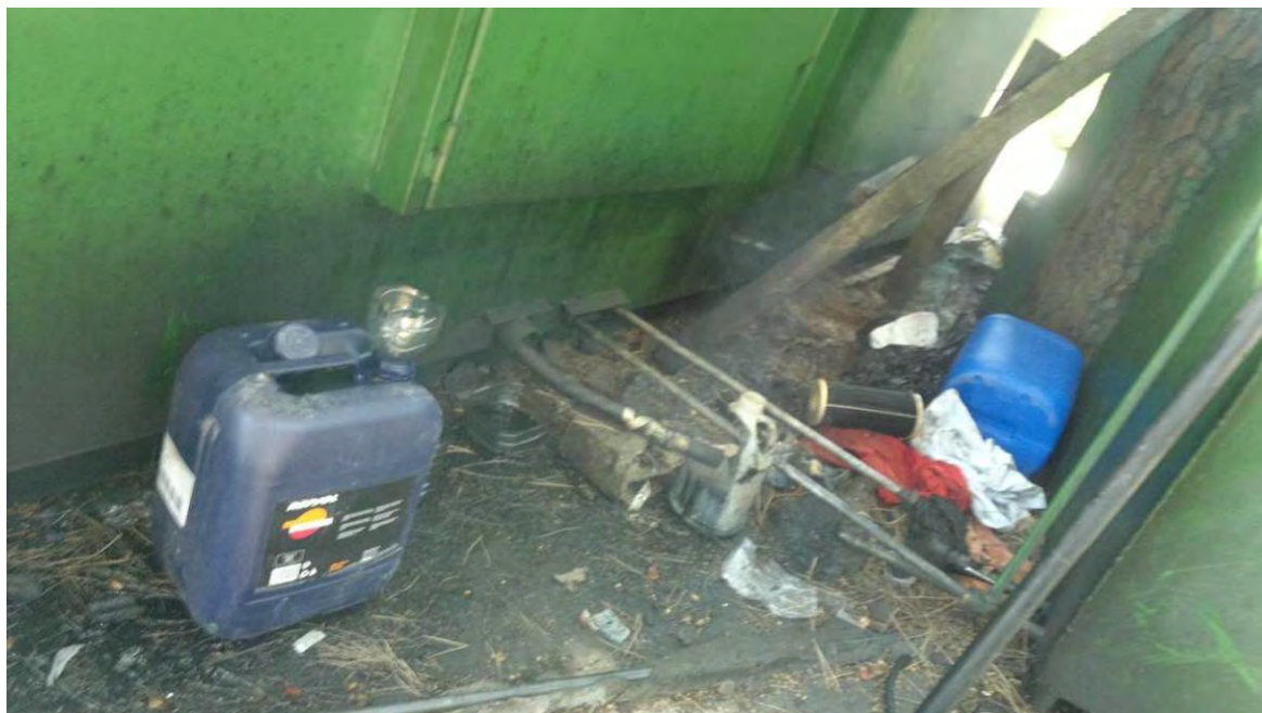
Figure 103: Surrounding of a generator used to sell electricity the public: oil spills, leakages and contaminated solid wastes
