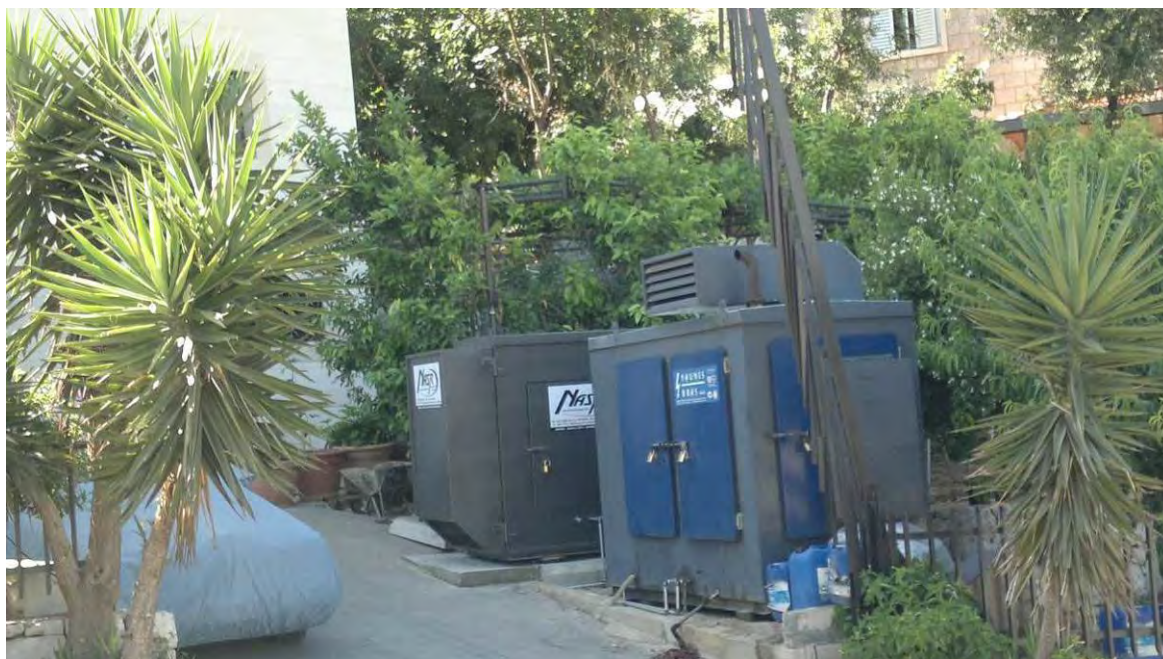
Figure 102: Well maintained private generator
