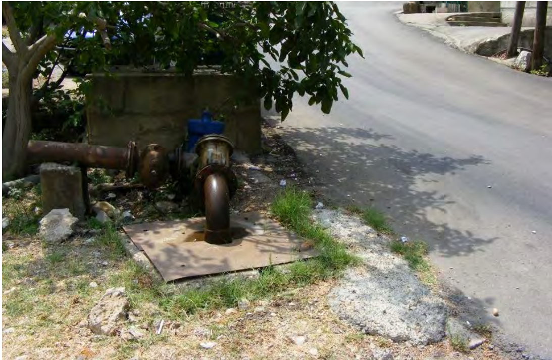
Figure 110: Drinking water well at Mokhada: without protection against contamination
