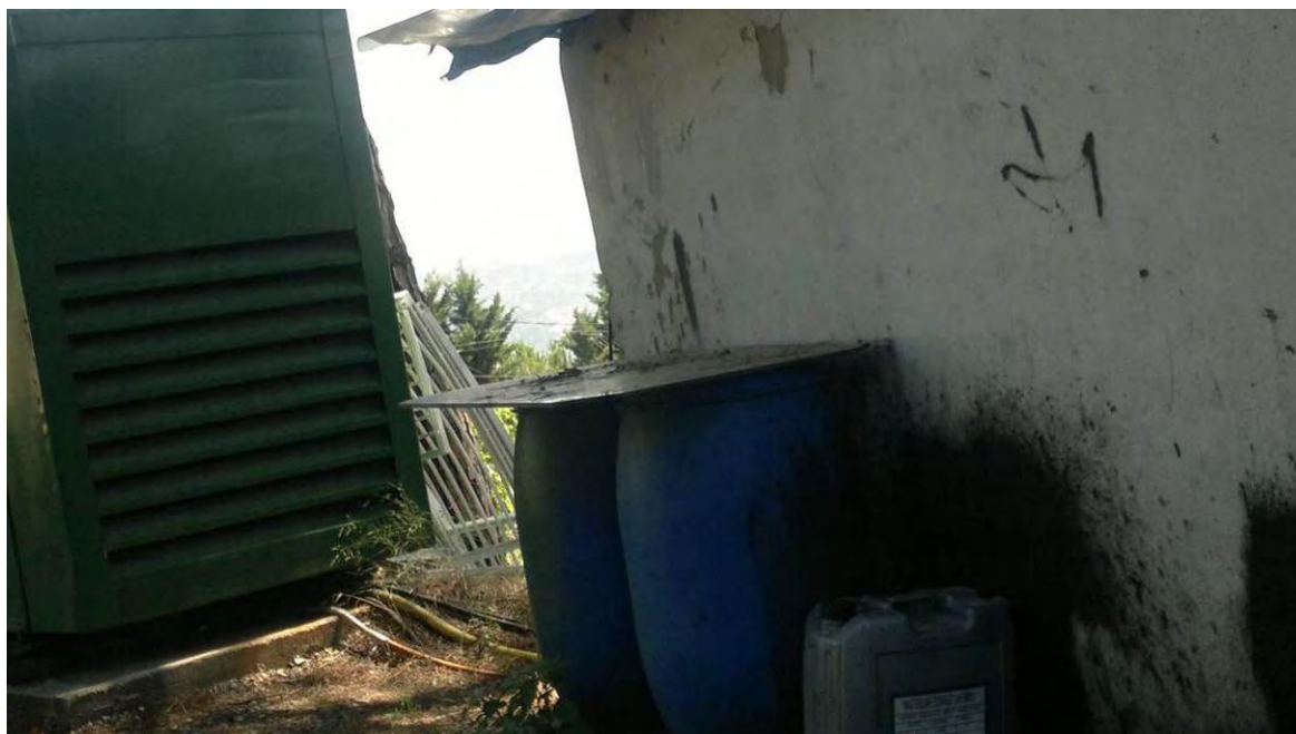
Figure 104: Improper storage of used oils at a generator dedicated to sell electricity to the public
