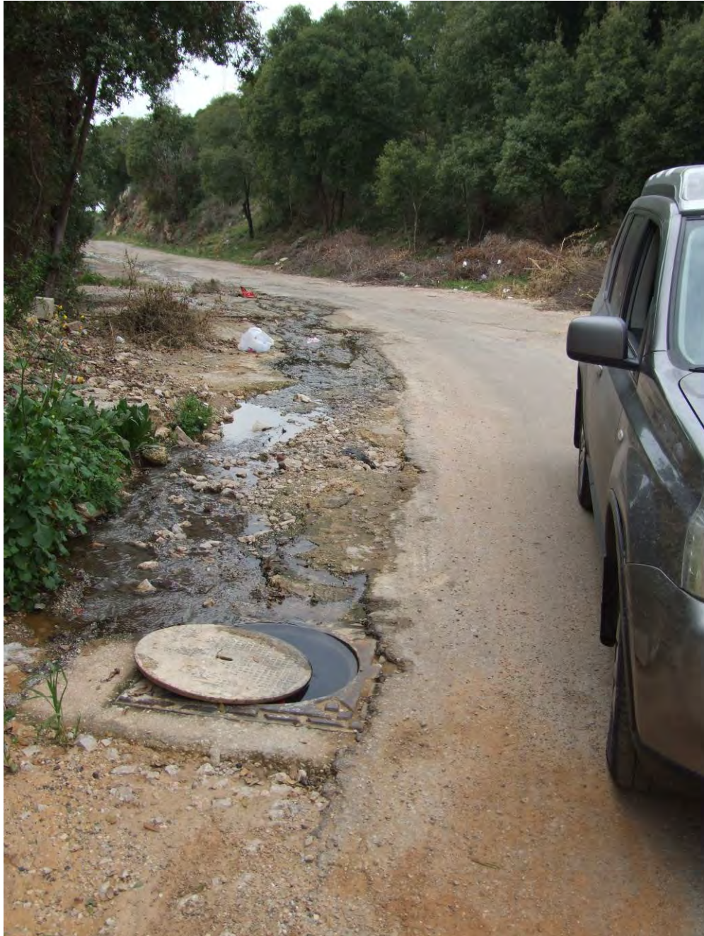
Figure 21: Flooding wastewater from septic municipal network in Ballouneh
