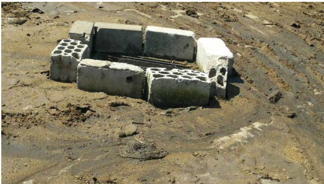
Figure 54: Drainage of liquid effluents generated by cleaning towards a bottomless open cesspit at the Ghosta slaughterhouse
