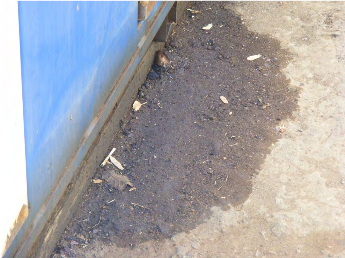
Figure 105: Diesel leakage from a generator
