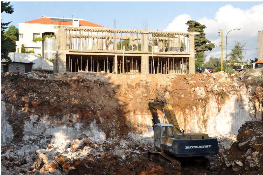
Figure 24: Excavated cesspit in highly karstified limestone
