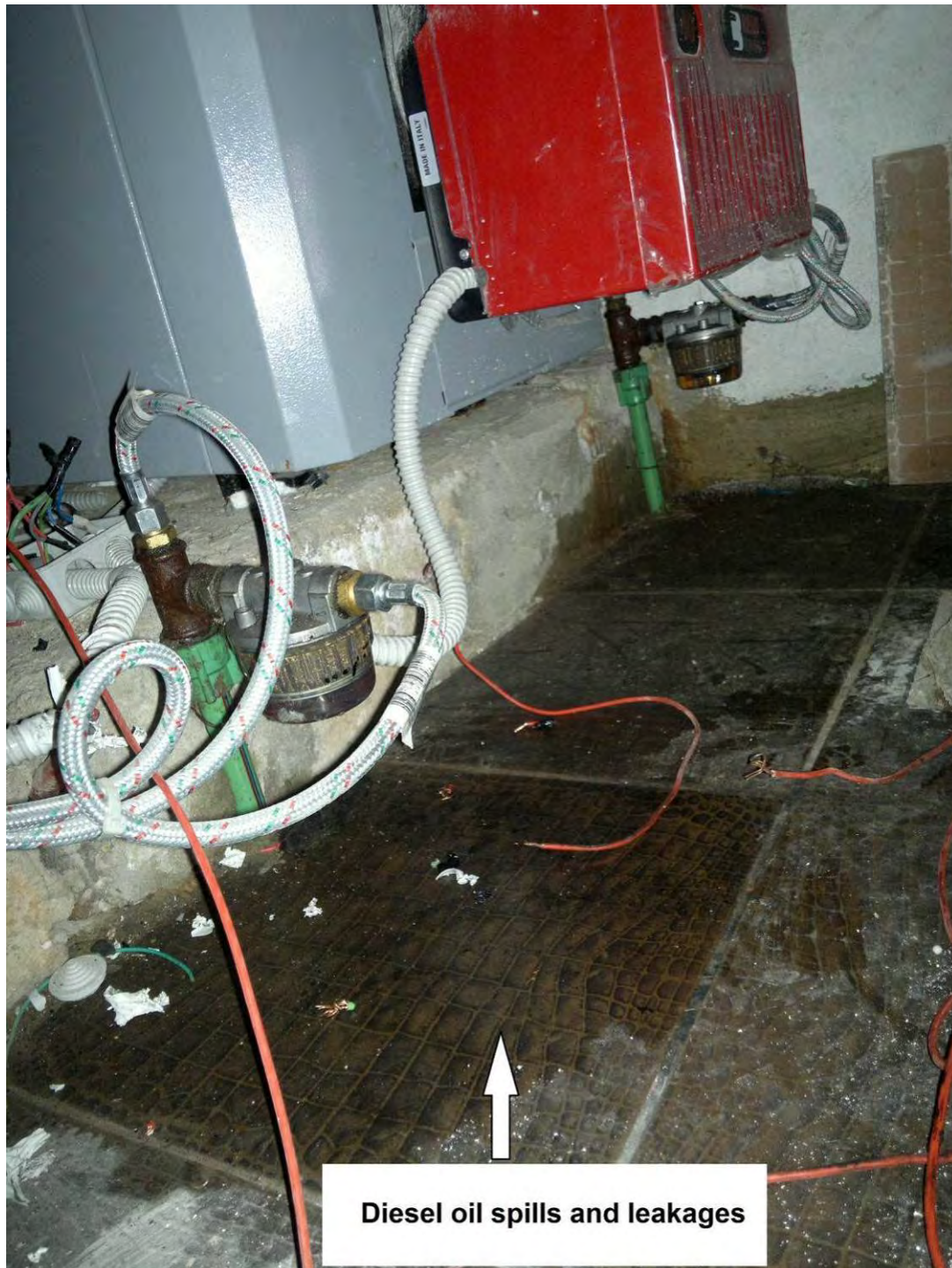
Figure 101: Leaking residential diesel heating system
