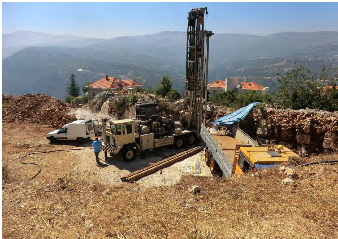
Figure 111: Private well drilled in July 2012 in Ballouneh for water supply to greenhouses directly over the underground river of Jeita
