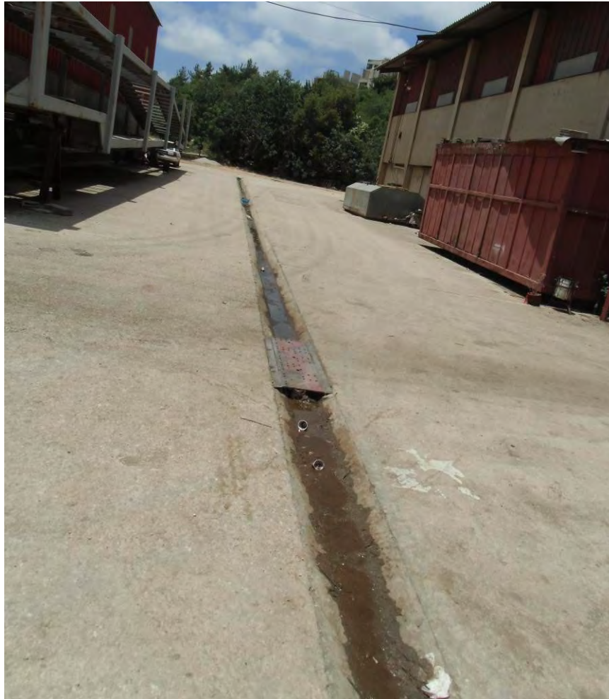
Figure 59: Drainage system discharging liquid effluents into the neighboring environment
