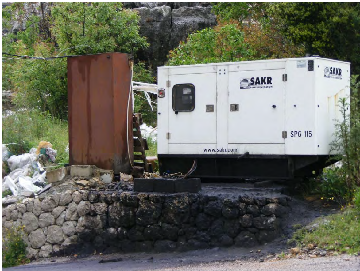
Figure 106: Oil and diesel spills surrounding a diesel generator in Ajaltoun
