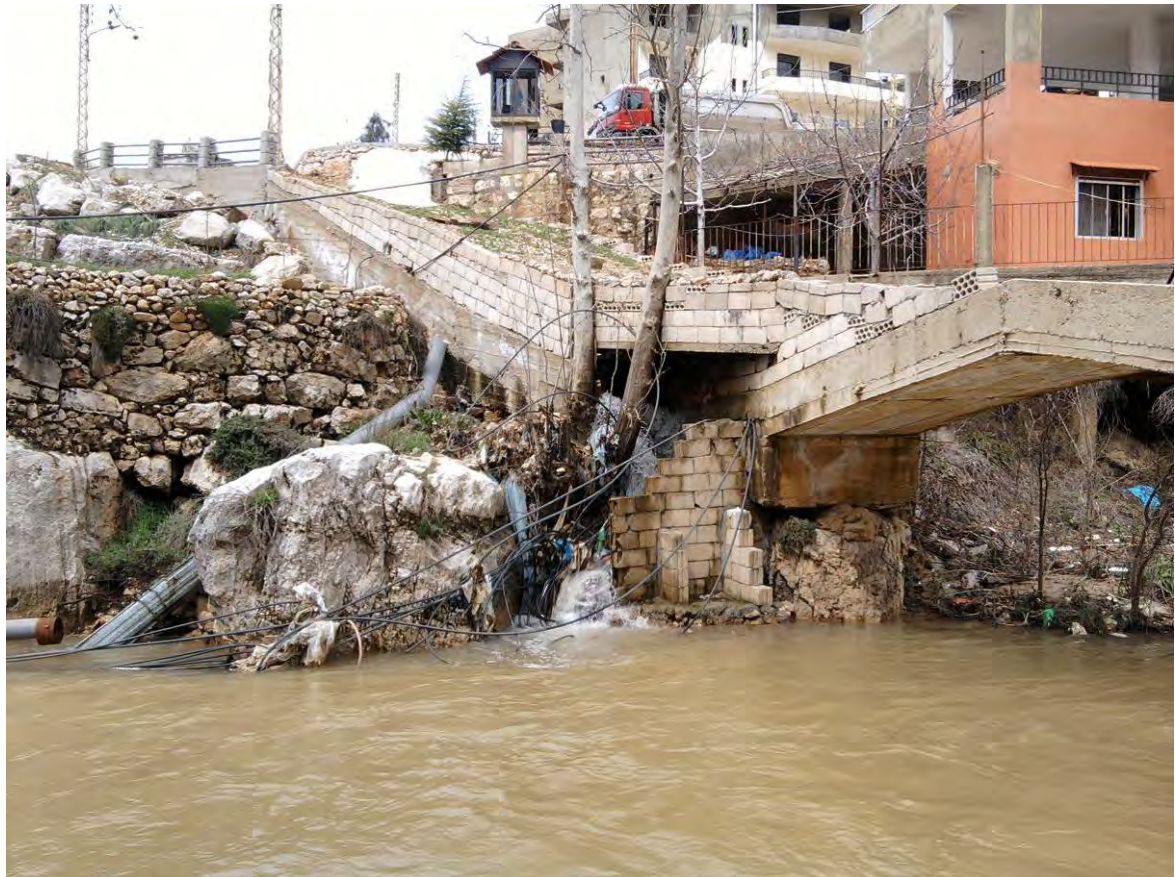
Figure 29: Sewage canal discharging into Nahr el Salib at Hrajel
