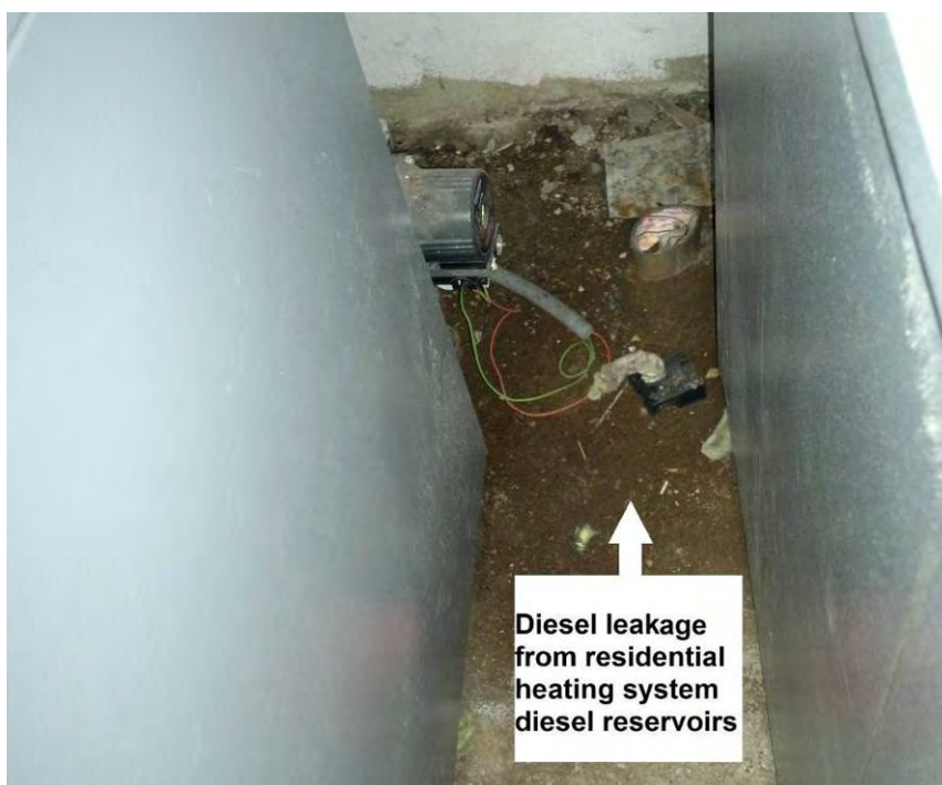
Figure 100: Observed diesel leakage from diesel reservoirs related to residential heating system at Raifoun
