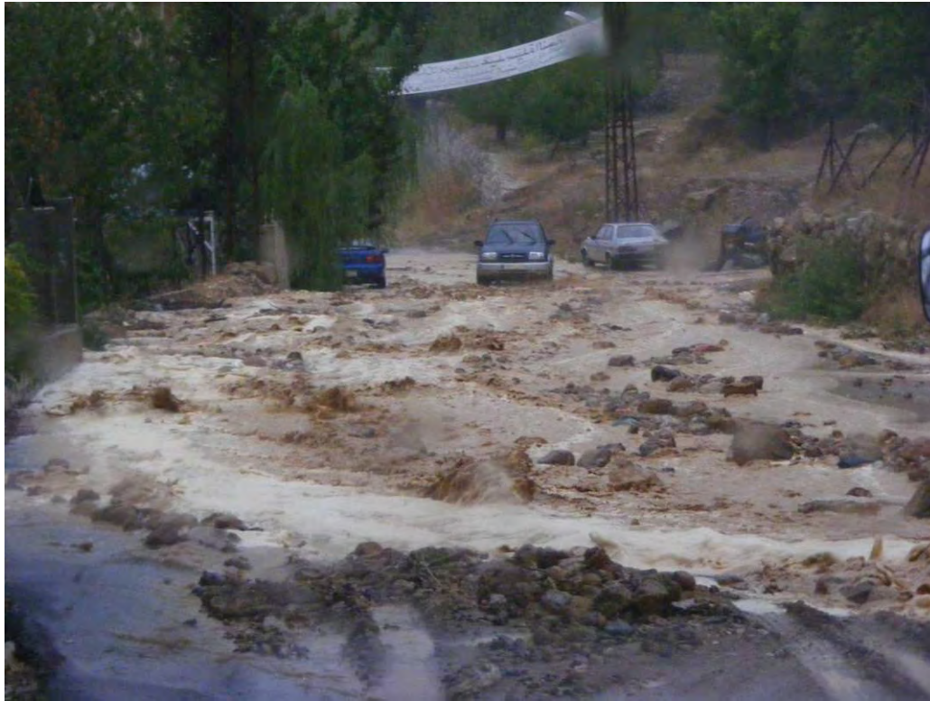
Figure 43: Rainwater flooding and damaging the road at Bqaaatouta during a rainy day
