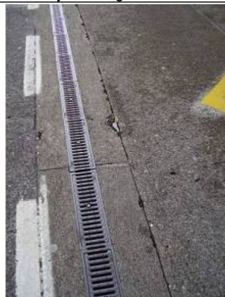
Damaged (leaking) joints along drainage channel
