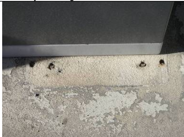
Holes for screw anchor not plugged!
