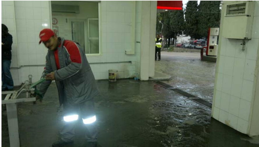
Photo 5: Gas station including a drainage system able to collect carwash waters. However, the laterers are conveyed to a hole leading to a leaking cesspit on the opposite side of the location.
