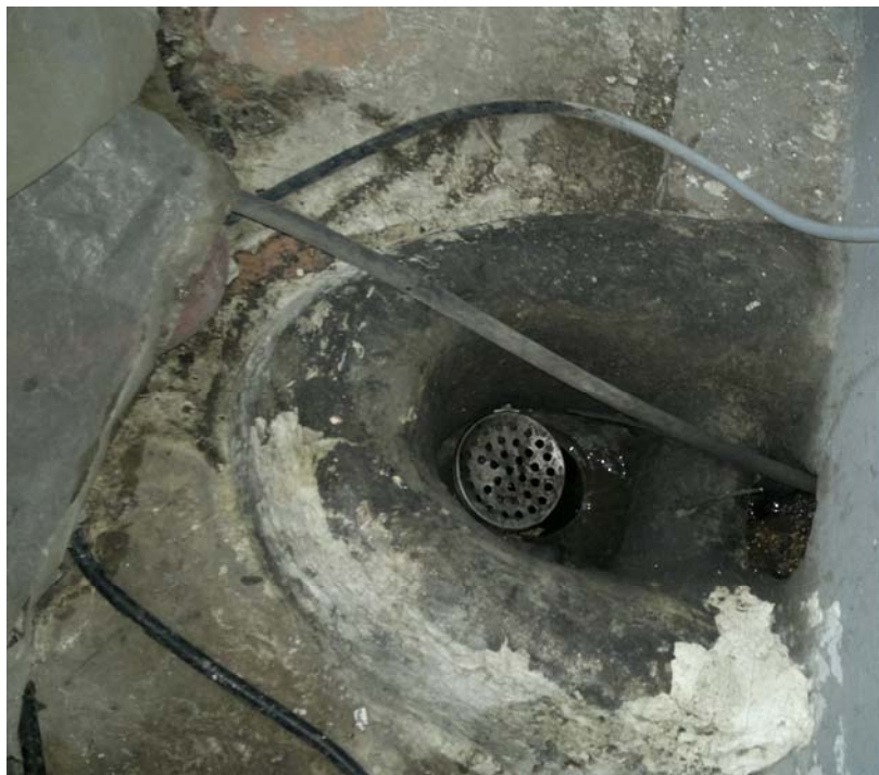
Photo 6: Hole in the wall and carwash waters flowing towards a cesspit instead of towards the existing separators.
