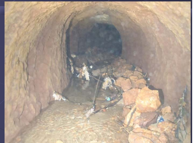
rock collapses in tunnel section
