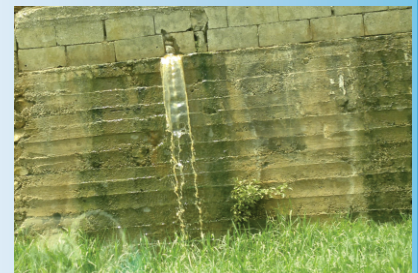
Discharge of slaughterhouse's effluent into the environment - without any treatment.
