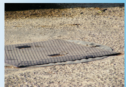
Improper closure of tank.
