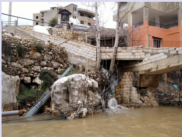
Discharge of untreated wastewater into Nahr es Salib
