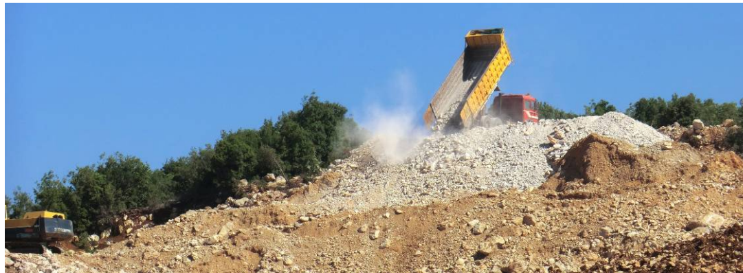
Figure 16: Construction Waste Dump at Mar Roukoz School
